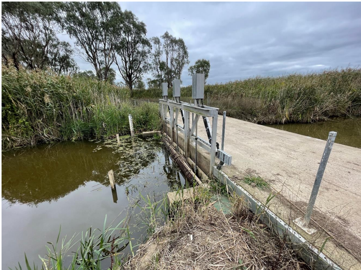
Figure 2-5 – inlet channel and penstock regulator (water level at time of image (21/04/23) was 1.0mAHD)
