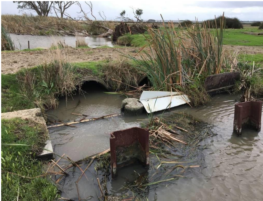
Figure 19. A section of the Hospital Swamps' watering infrastructure at the bottom of the barge hole in the inlet channel. Flow controlled by placement of wooden boards in concrete grooves (S.Blum-Caon, 2019)
