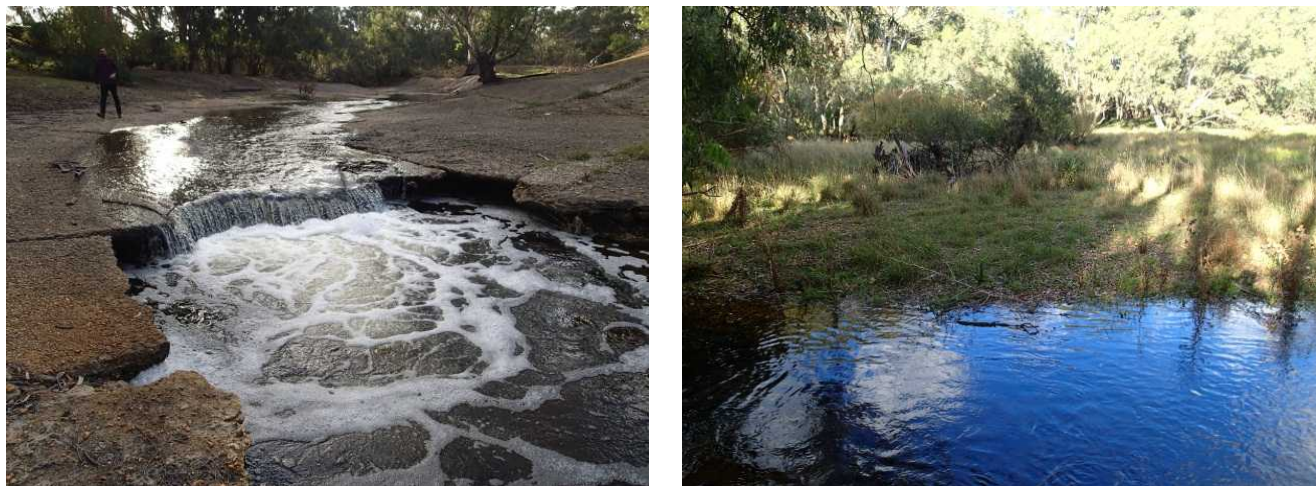
Figure 5.8: Photographs of Moorabool River diversion downstream of Batesford adjacent to limestone quarry. Cracking and erosion of concrete channel lining works (left photo). Large sediment slug filling valley and creation of shallow flow conditions (right).
