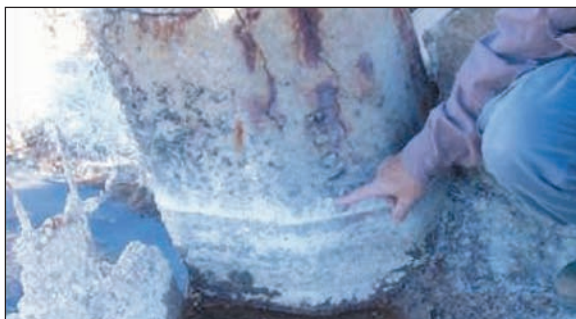
Fig. 8: Concrete pipe has eroded due to the action of sulfuric acid released from ASS.
